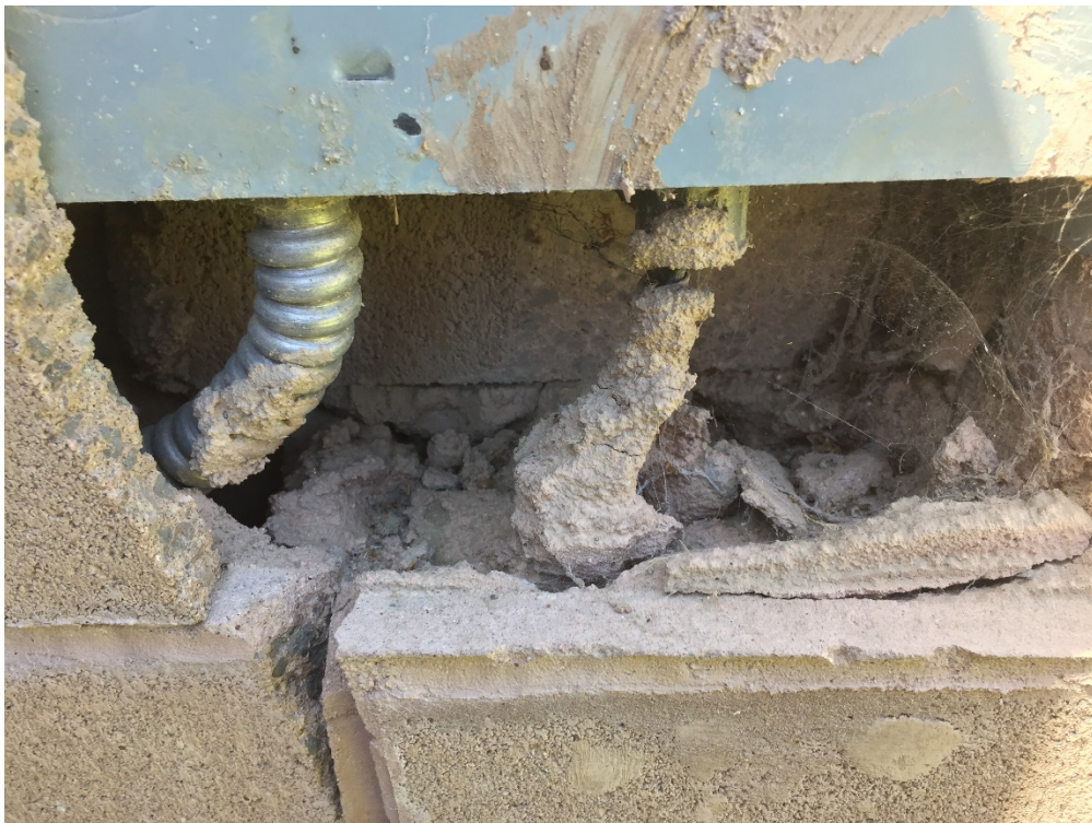
Block wall in resident's yard on Monterey Lane
